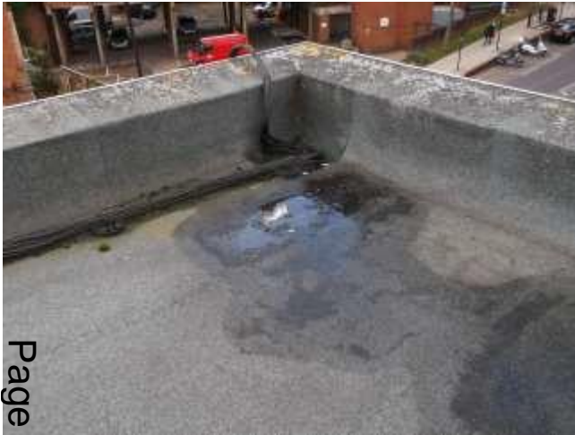
Above: Mineral felt flat roof in reasonable condition for its age requiring some repairs and cleaning off and resealing of outlets.
